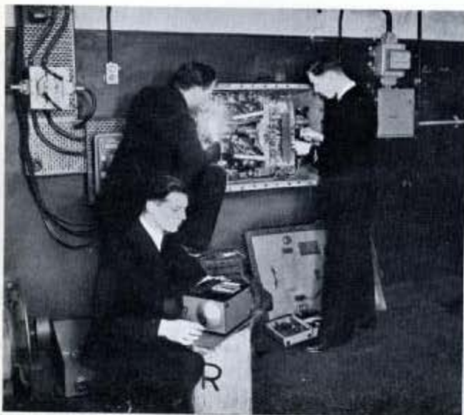
Fig. 47—Electrical Artificers spend 4 and 6 weeks respectively, during their F and G Class periods, in the Electrical Demonstration Room; here they are shown carrying out tests on a ring main breaker which is part of a ship's electrical installation.
