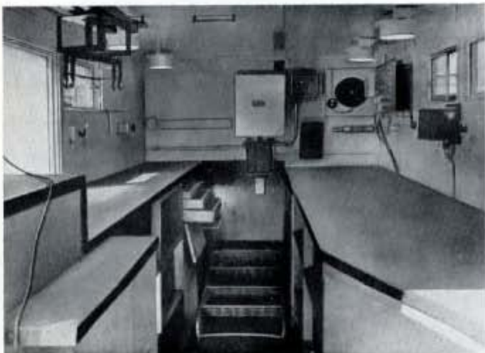
Fig. 327—An interior view of one of the Radar Workshops of the M.A.R. Component; the metal steps used for entering the workshop when mounted on the lorry chassis, can be seen lying on the floor.
